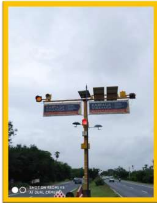
Solar powered traffic signal at the entrance of college
